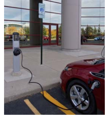
Charging Station at Magna E-Car
