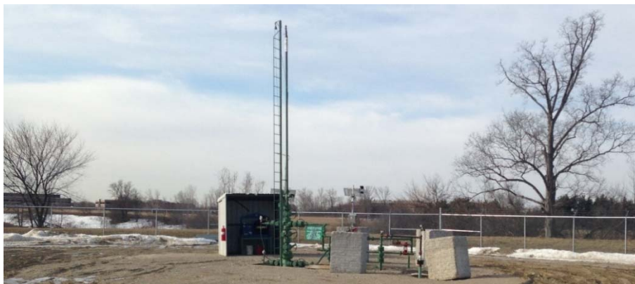
In typical Auburn Hills’ fashion, the Planning Commission didn’t just write an ordinance for gas and oil drilling ... many experienced it
